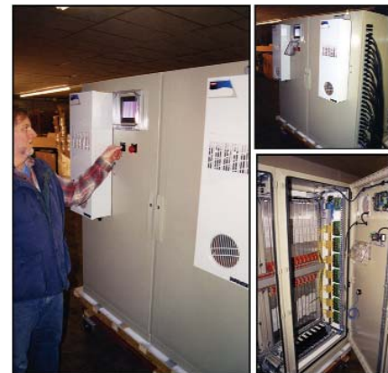
EA Engineer performing a final inspection on a 9,300 Watt Open-Channel UV prior to shipping to Montana Fish, Wildlife & Parks, Fort Peck Hatchery
